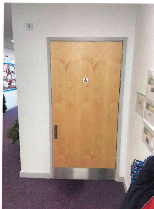
This is the Year 5 and 6 disabled toilet. There is also a disabled toilet for Year 3 and 4, and one in the Reception area for Key Stage One.
